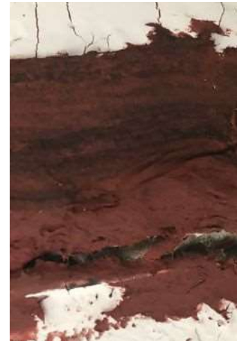
Movement issues found at an existing head of wall. Corey Zussman photo.
