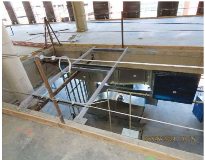
Photo of elevator shaft, which the shaftwall needs to be coordinated to be properly supported. Corey Zussman photo
