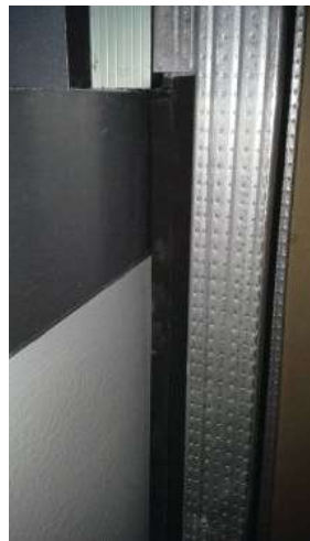
Photo of firewall and curtainwall joint that allows for lateral movement. Corey Zussman Photo
